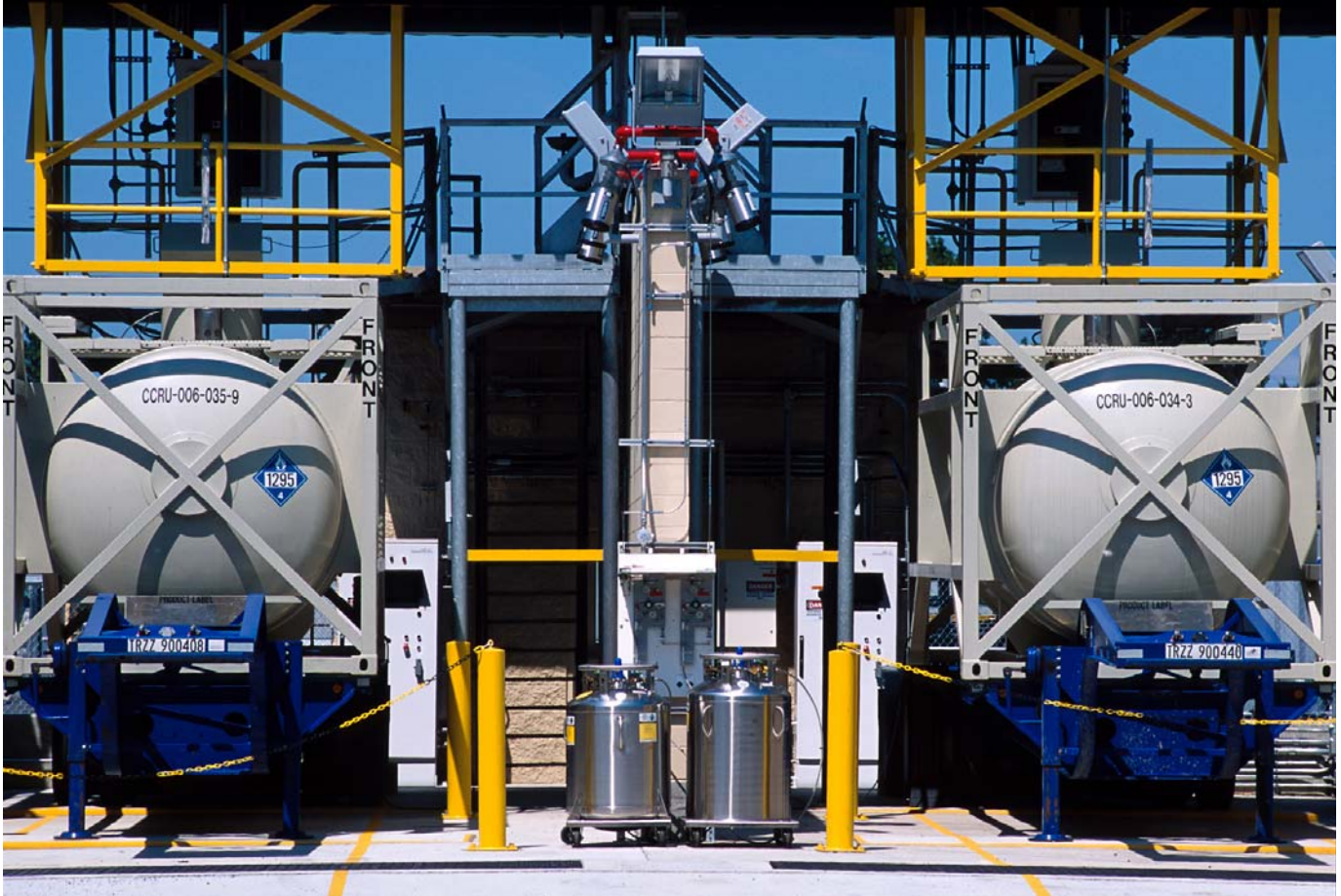
Fig 1 Dual ISO module Tanker Installation Shows Level of Complexity for BSGS
